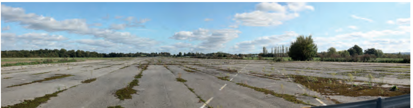
View towards eastern extent of runway from central section (Junction of FP13 & FP15)
